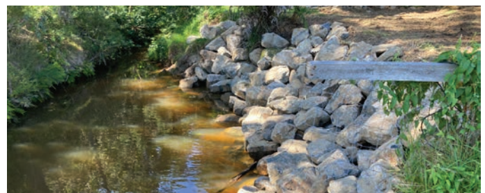
A rock revetment put in to protect a section of the Wahitapu Stream bank from eroding.
