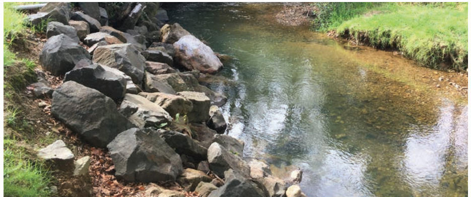
Rock rip rap protects the Karaka Stream bank from erosion on a bend.
