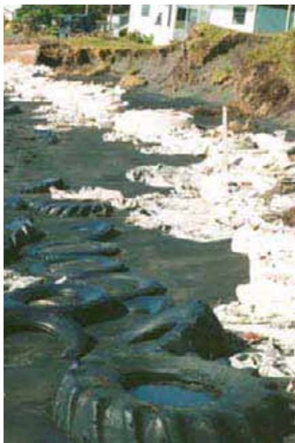
Coastal erosion at Aotea on the west coast, 2002
