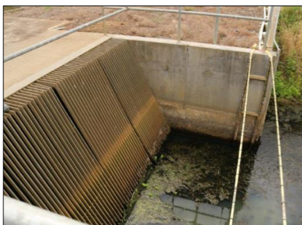
Figure 10: Pump station inlet debris screen. White pipes are PIT antennae
